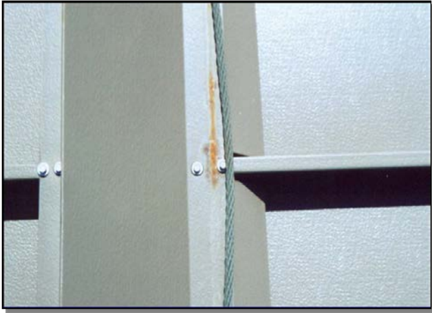
Figure 3-13 New Roof Corrosion from Direct Contact with Electrical Conductor
