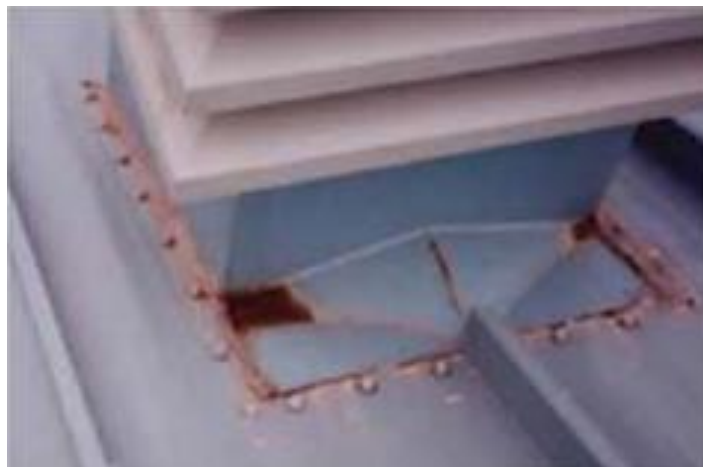
Figure 2: This galvanized curb has already started rusting at the welds in less than one year
