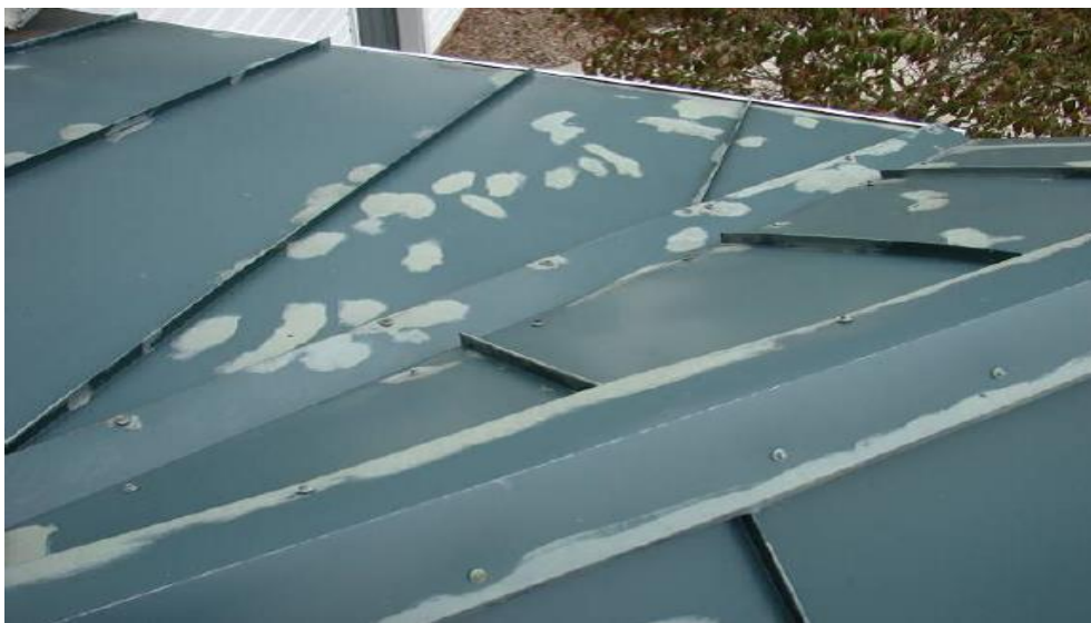
Figure 1 - Appearance of a pre-coated metal roofing where a low performance field applied air-dry paint system was used
