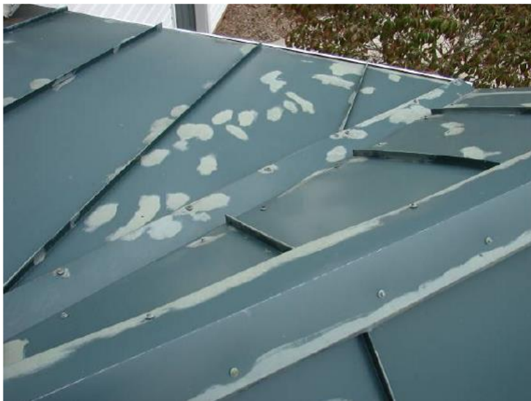
Figure 1 - Appearance of a pre-coated metal roofing where a low performance field applied air-dry paint system was used
