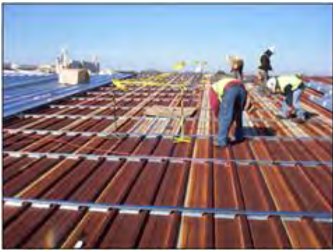
Factory-notched structural sub-purlins being installed over old aging roof and receiving a new traoidal standing seam roof (Photo courtesy of Roof Hugger, LLC)
