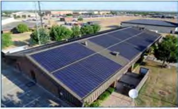
Photo 8-5: Thin-film Surface Mounted Laminate PV (Courtesy of Metal Sales MFG.)
