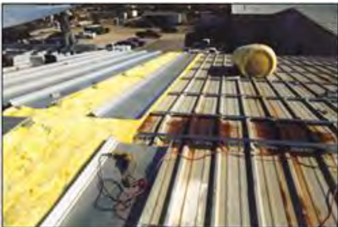
MOM assembly being installed with unfaced fiberglass insulation (Photo courtesy of Roof Hugger, LLC)
