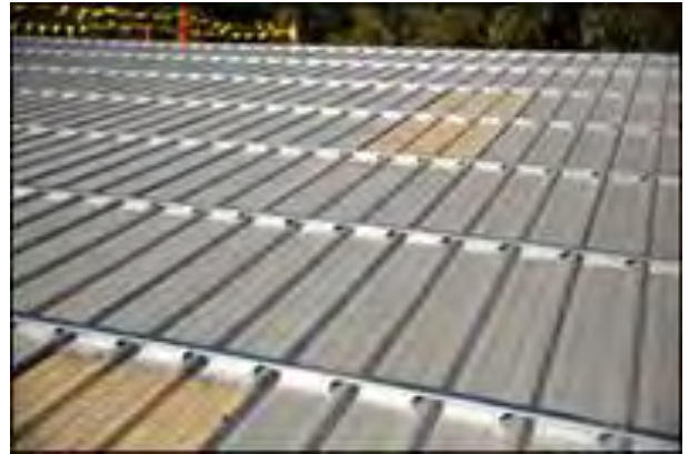
Photo 4-2: Existing exposed fastener that has failed receiving new factory-notched sub-framing for a new metal roof to be installed (Courtesy of RetroSpec, LLC)
