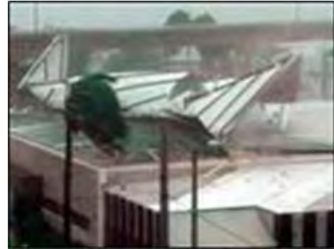
Photo 3-3: Hurricane force wind on metal retrofit (Courtesy of RetroSpec, LLC)
