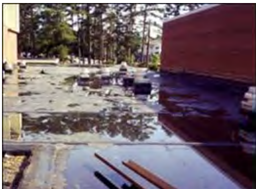
Photo 3-1: Ponded water on flat roof (Courtesy of Retrospec, LLC)
