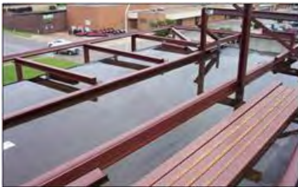
Photo 5-4: Existing flat roof flooded after a rainfall due to continuous base members not being shimmed at their point of attachment. (Photo courtesy of retrospect, LLC)
