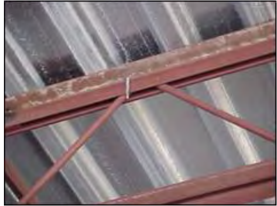
Photo 4-1 – Existing Bar Joist with retrofit framing base member anchor showing at top chord (Courtesy of retrospect, LLC)
