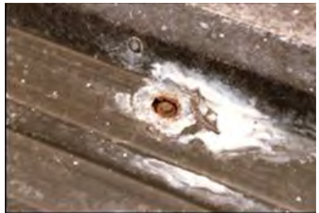
Photo 4-3: Existing exposed fastener that has failed due to movement over the years (Courtesy of RetroSpec, LLC)
