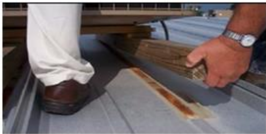
Figure 3. Roof corrosion from treated wood
