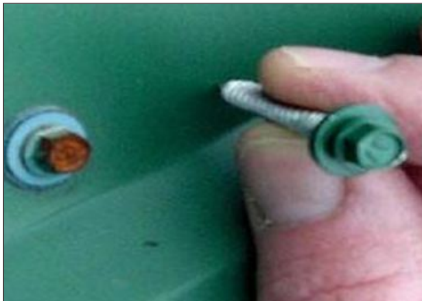
Figure 14-31 Correct Fastener Compared to Installed Fastener
