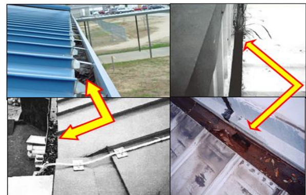
Figure 19-9 Gutters Need Cleaned and Inspected Regularly
