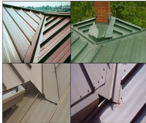
Figure 19-13 Valley Issues Affect Water Flow and Drainage
