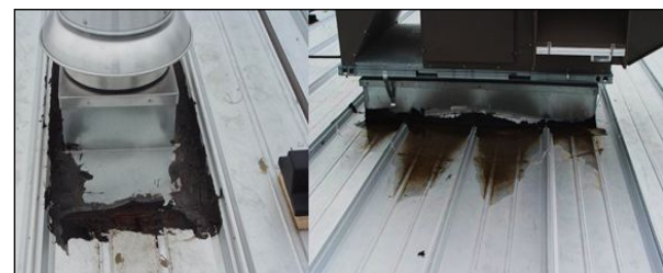
Figure 8-9 Improper Curb Types
