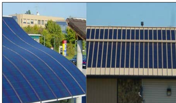
Figure 8-34 Photovoltaic Laminate on a Metal Roof
