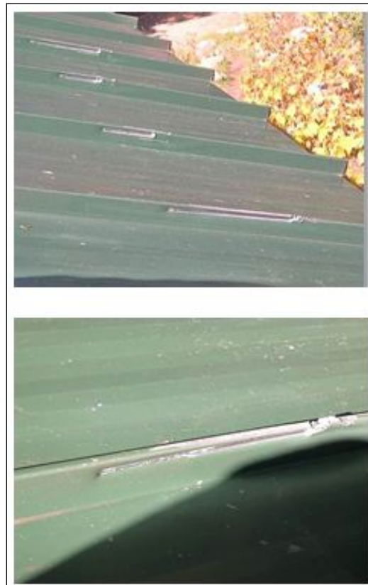
Figure 8-24 Roof Damage from Improper Installation
