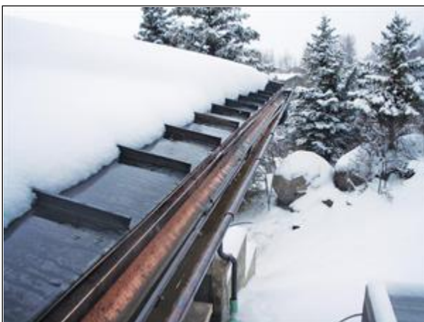
Figure 8-21 Electrical Ice Melt System Installed Along the Fascia Avoids Penetration of the Roof Surface
