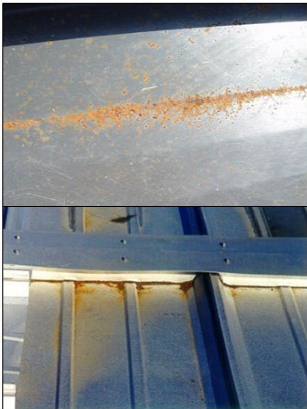
Figure 16-32 Failure to Remove Cutting Debris (Swarf) Quickly Causes Panel Corrosion and Rust
