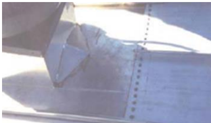
Figure 6: This curb has 12” of clearance between the panel ends and the water diverter, which prevents water buildup.
