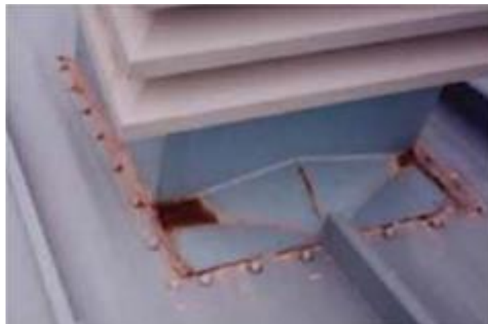
Figure 2: This galvanized curb has already started rusting at the welds in less than one year
