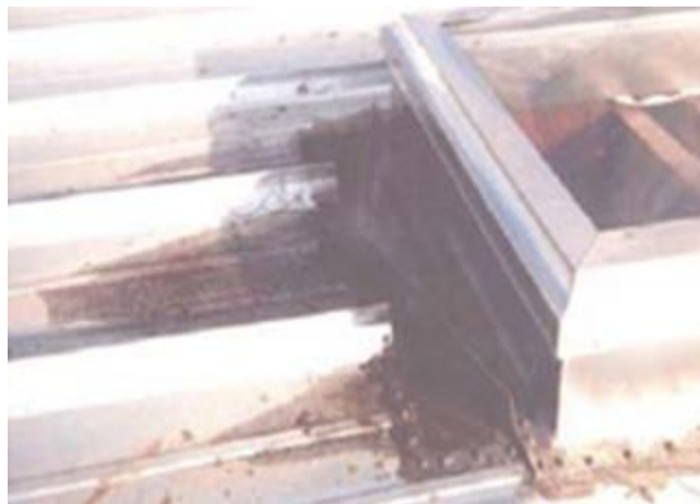
Figure 9: Curb with inadequate clearance on the upslope end allows a water head to build up
