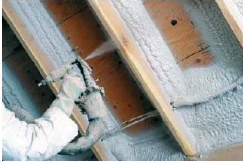
Photo of SPF being applied to wood deck using picture framing technique. Spraying foam onto a metal panel surface would be done in the same fashion. (Courtesy of Spray Foam Professional Magazine)
